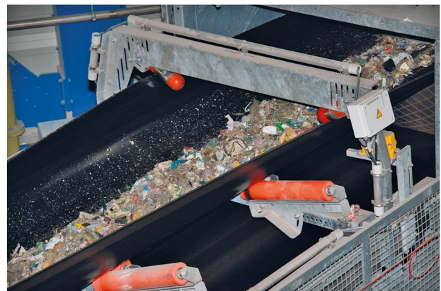
Pipe conveyor with pre-treated input fuel, before closure of pipe (© Linz Strom GmbH)
