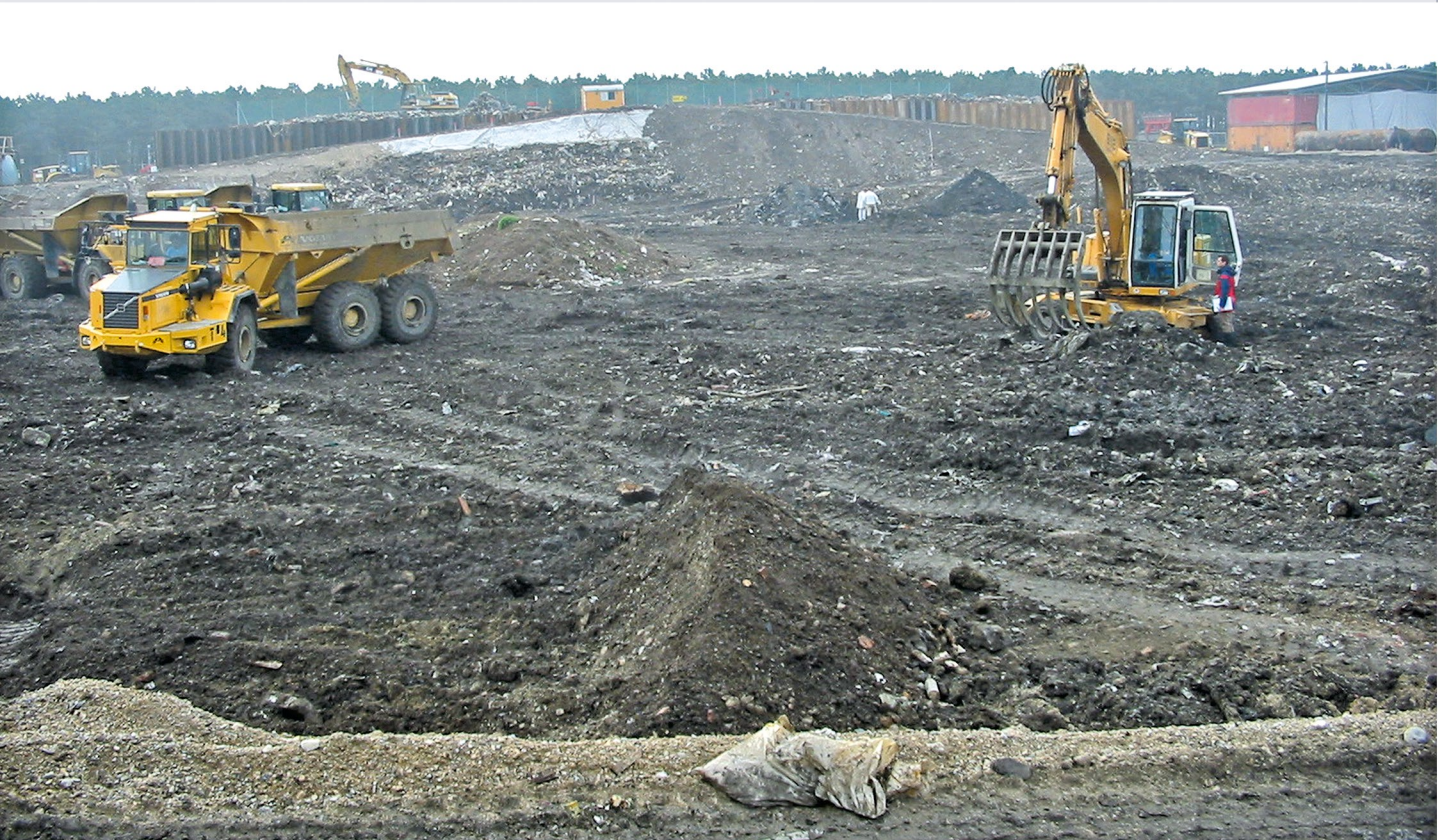
Excavation of waste materials (mainly domestic waste), contaminated soil, and barrels filled with waste solvents (© UVP GmbH)
