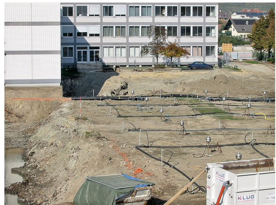
Aerobic treatment to reduce content of methane in nearby buildings (© UVP GmbH)
